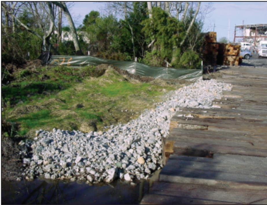
Rip-rap (rock) was used to filter runoff and control erosion near the trestles.
